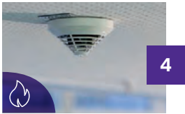
Fire Alarm Systems
